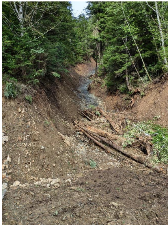
B: Copper Ridge Landslide, Point 1021, Middle Zone conditions with steep colluvial slopes.
