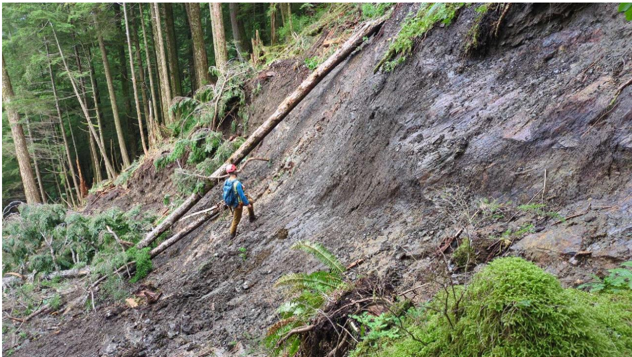
B: 3rd Avenue Landslide, Point 15, east side of headscarp looking north.
