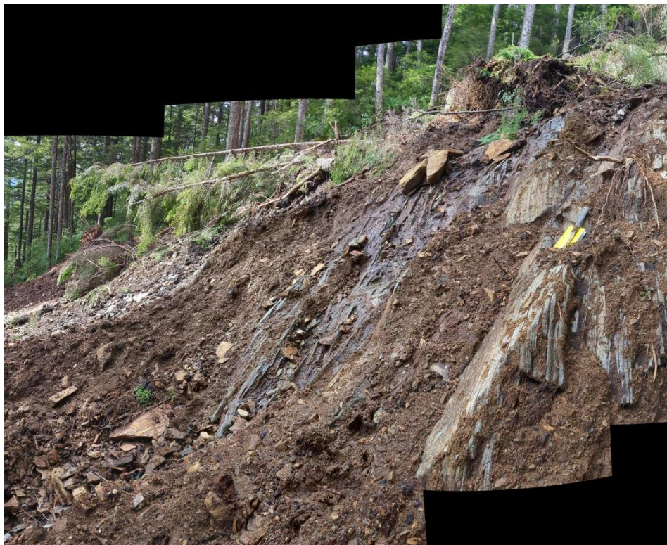
B: Copper Ridge Landslide, Point 1038, Upper Zone, headscarp conditions with phyllite bedrock exposures, looking northwest.
