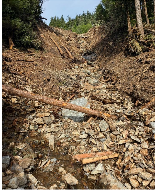
A: Copper Ridge Landslide, Point 1050, Lower Zone, steep slope below access driveway switchback.
