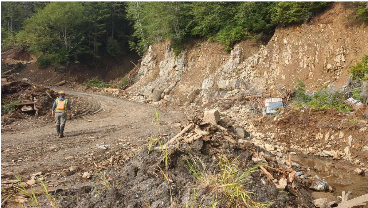
B: Copper Ridge Landslide, Point 1022, Lower Zone, stream channel diversion adjacent to access driveway switchback looking southwest.
