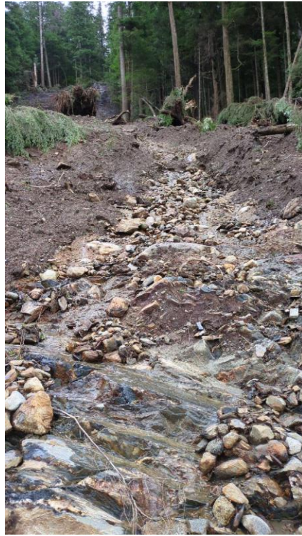
A: 3rd Avenue Landslide, Point 5, phyllite exposure in recently developed drainage channel.
