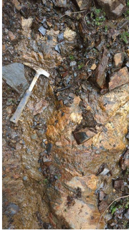
A: 3rd Avenue Landslide, Point 26, glacial till exposure.
