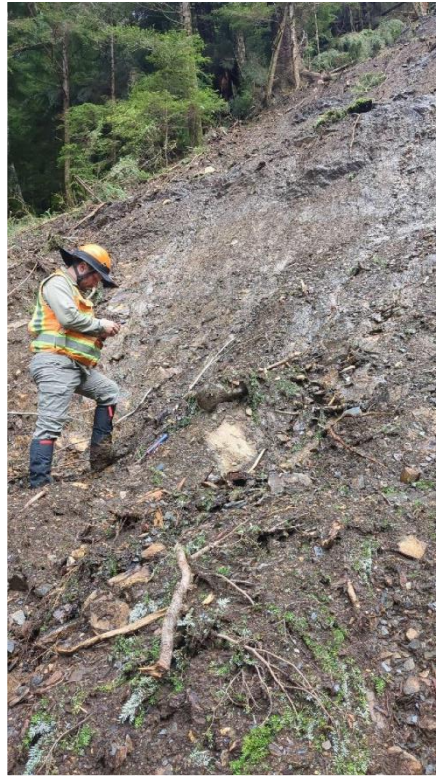
A: 3rd Avenue Landslide, Point 5, phyllite exposure below headscarp with unfavorable jointing.
