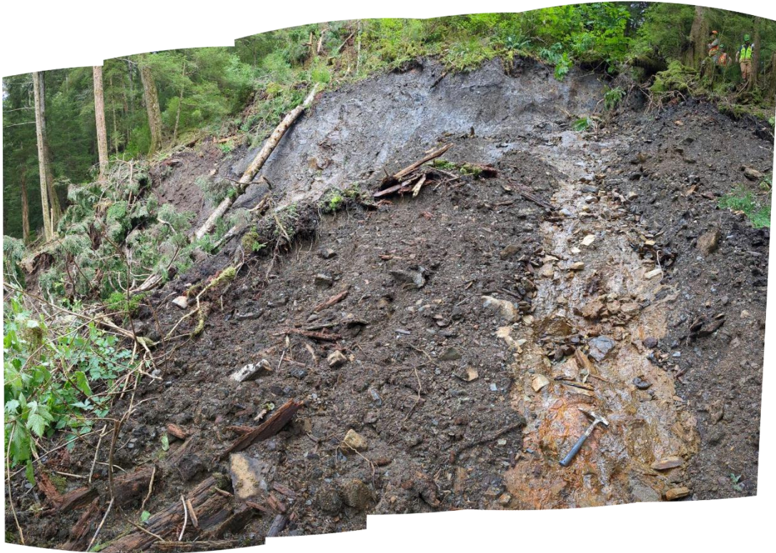
A: 3rd Avenue Landslide, Point 15, middle portion of headscarp looking upslope to northeast.
